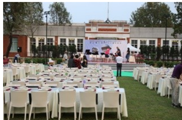
Saturday daytime electrical wiring/sound, and table settings preparations in the front lawn, gala dinner vicinity.
