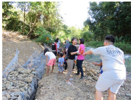
Christopher Liaw (Senior) and Jade R. Justin (Sophomore) work on the gabion in the heat and humidity of Mindoro Island
