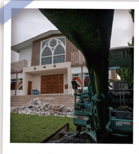
Bayview Church / King Huy Hall road being repaved in the northeast section of the Clear Water Bay campus.
