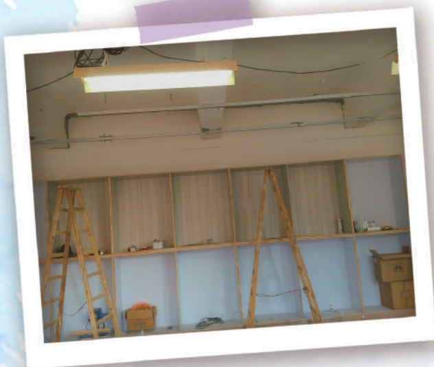
The new wall shelving unit being put in place by ladders in the classroom
