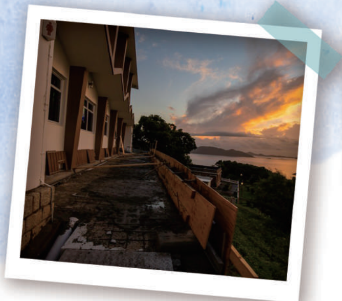
Rear patio view of Bayview Church / King Huy Hall during the second renovation phase.
