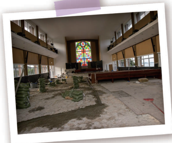
Following the 31 July 2020 board approval, Bayview Church / King Huy Hall received repaired and refinished pews, a vinyl plank to replace termite-prone teak wood flooring, a new air conditioning system, new outdoor floor tiles on the rear patio, and granite fencing to replace the prior iron fencing.
