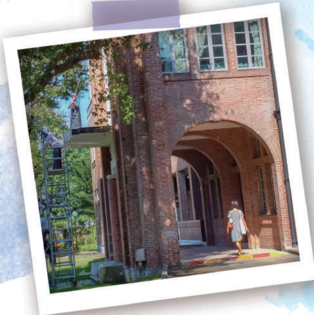
Alice walks under the HKAC Admin. Building's archway, as workers repair the facade
