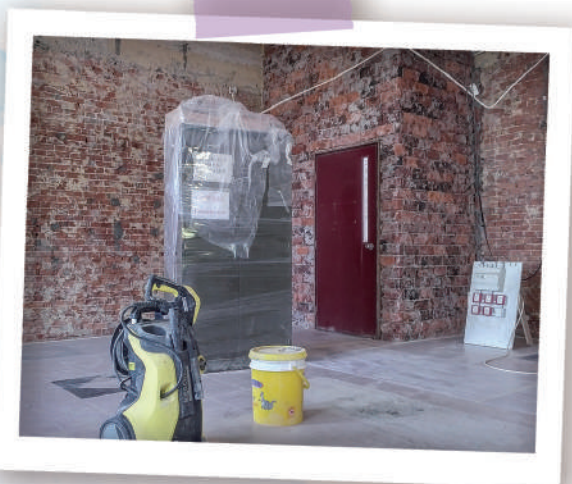
Brickwork exposed after wall paint removed. Old wiring, plastic shrink-wrapped new cabinet door. Yellow bucket and renovation machine tool are on the foreground
