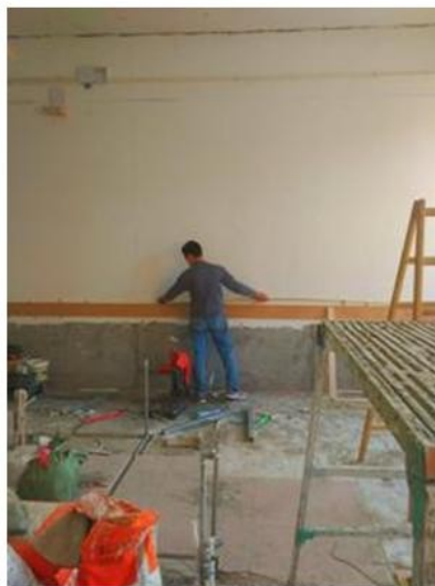
Laying down new wiring on back wall inside the Biology Lab classroom
