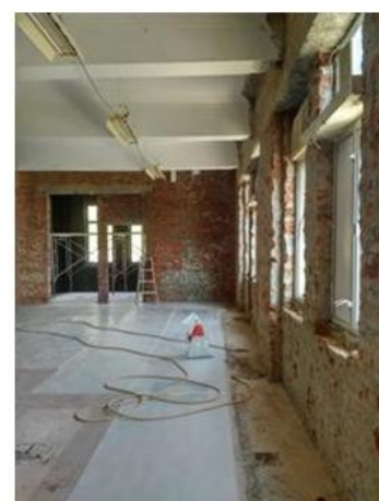
Electrical cords meander on the floor of the Chemistry Lab. Right side and inner room windows are shown. Interior brickwork is exposed at the doorway to the interior room chamber.
