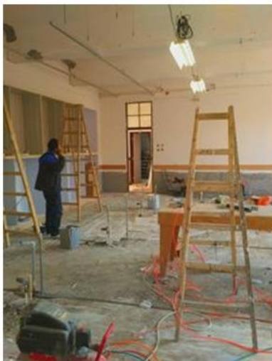
A worker in the Biology Lab is about to continue with renovation activity
