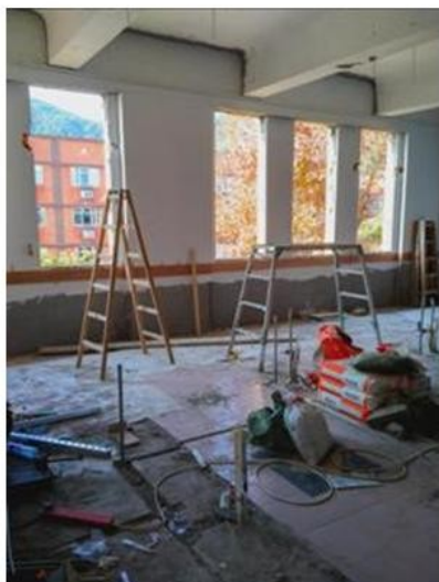
Re-plastering materials and ladders inside the Biology Lab classroom with views of the dormitories and High Junk Peak in the background
