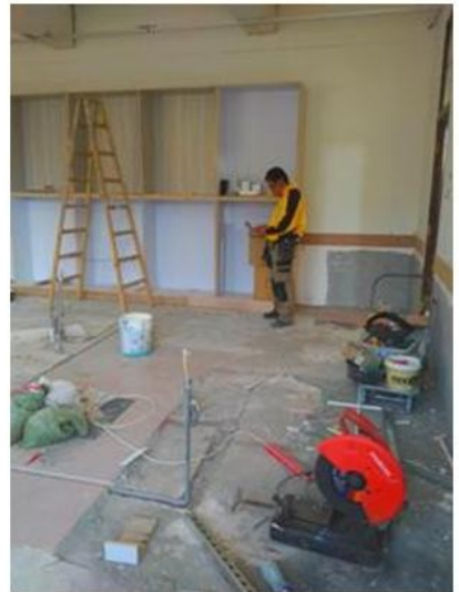
A worker in the HKAC Biology Lab is about to continue renovation activity.
