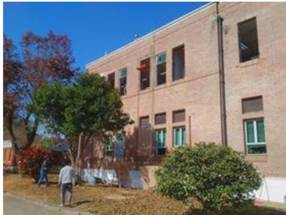
Workers about to climb ladder to spray clean the exterior bricks of the Biology Lab
