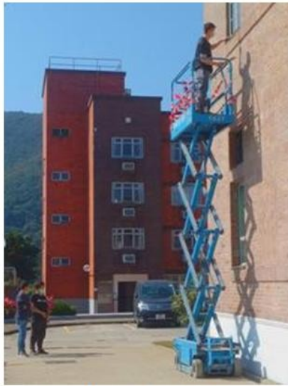
A worker adds grout sealant to the HKAC Biology Lab window sill.
