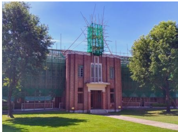
The rooftop spire of the HKAC Administration Building is all covered in a green mesh construction netting.
