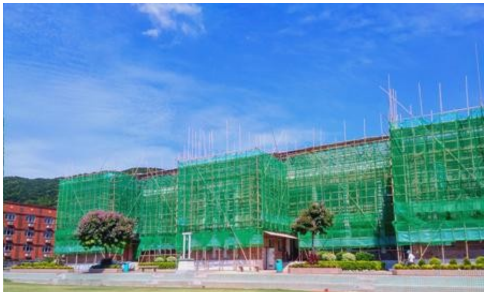
Kelly green mesh netting covers the bamboo scaffolding on the reverse façade of the HKAC Admin. building
