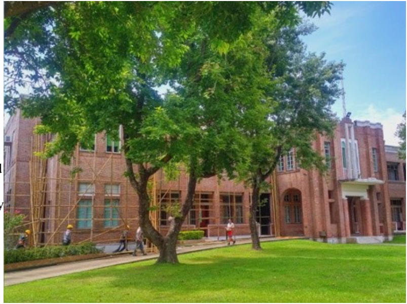
Front façade of the HKAC Administration building with bamboo scaffolding being erected by workmen in yellow construction hats.
